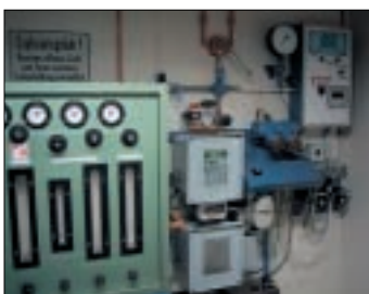
Equipment for mixing and monitoring the gas-air mixture
